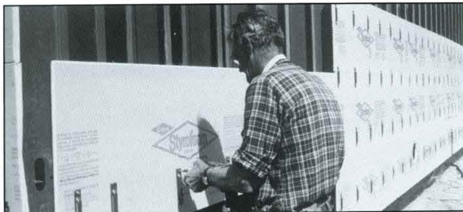
The insulation installation is a one-step job, completed at the same time that the brick ties are installed. The tongue-and-groove edges fit together snugly, helping to reduce air infiltration.
