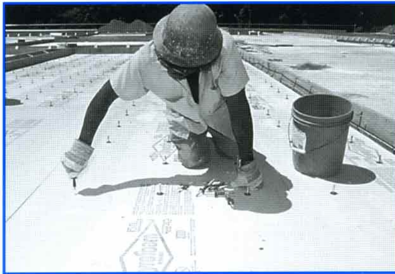
Pre-drilled STYROFOAM brand insulation is placed over fresh concrete, then fiber composite connectors are inserted into the insulation by hand to ensure the fluid concrete flows into the notch in the bottom side of the connector.
